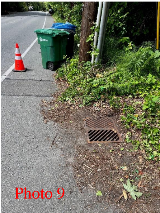
Photo 8 shows the structure redirecting the SE Maker system north along SE Mercer Way. The system is relatively flat and has an 18" diameter. GIS mapping shows a surface drainage feature draining to this location. There are no signs that this feature exists.
